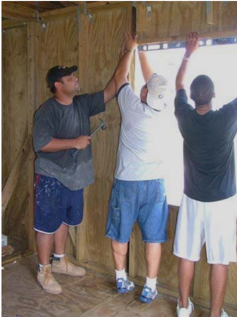
A Group of Public Works employees install windows to help speed up Mr. Hooker's recovery process.
